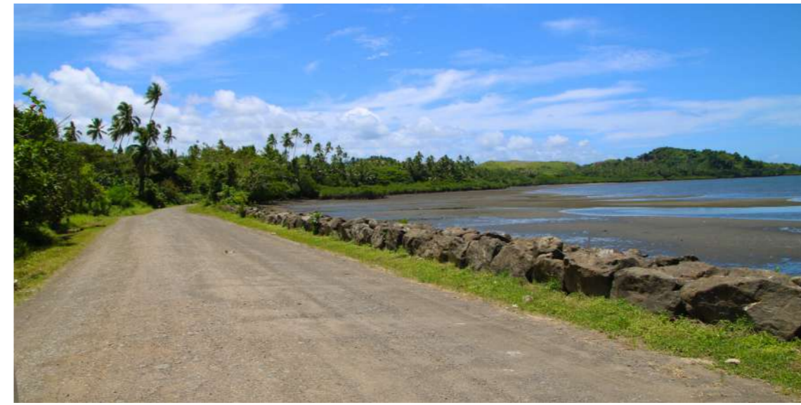
Coastal protection works along a section of Natewa West Coast Road in Vuinadi Village.
