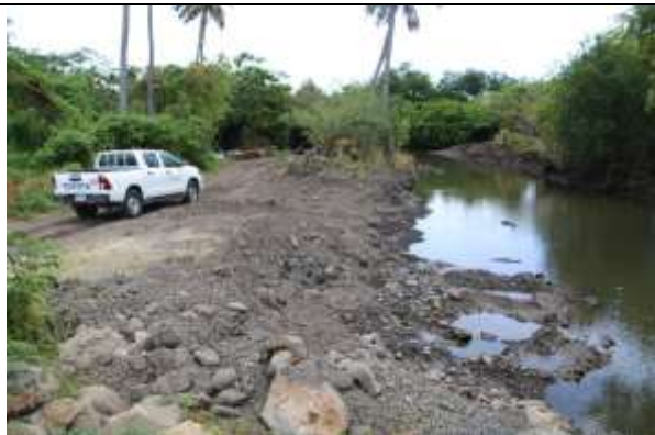
Figure 11: Navutu Section of sedimentation build-up that was rectified.
