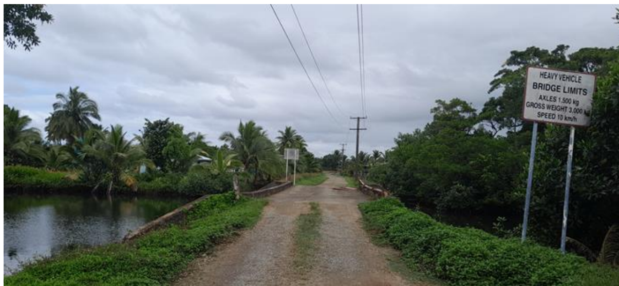
Namelimeli Bridge in Navua is closed to all vehicles.
