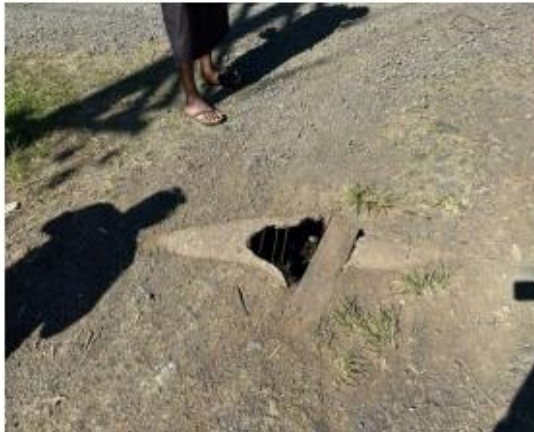
Figure 4: Damaged culvert at a residential access.
