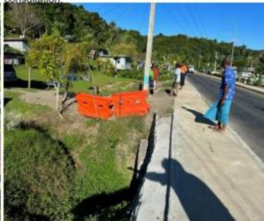
Figure 5: Trench too high, request to install guardrails.
