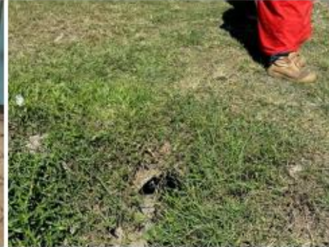
Figure 3: Damaged Culvert at a village access.
