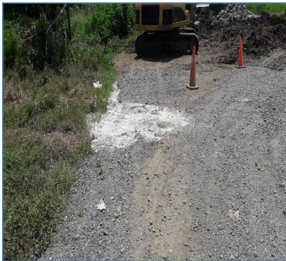
Photo 3 – Spilled cement on the road.
