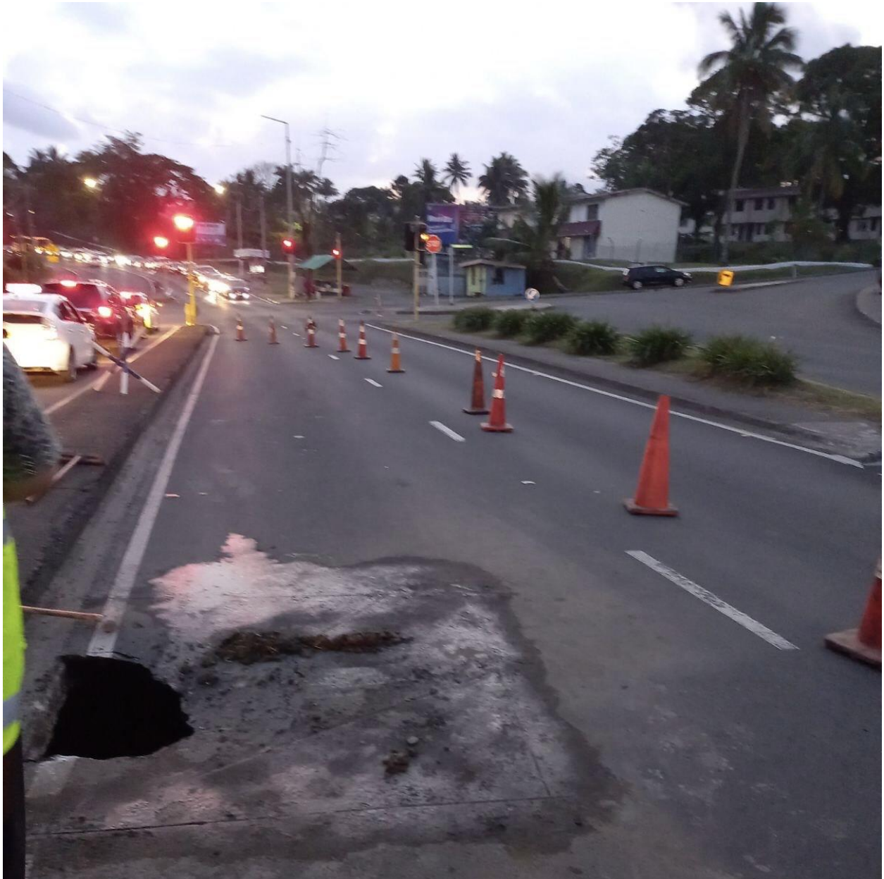
Picture Caption: Sinkhole on Kings Road near the 4miles Bridge.
