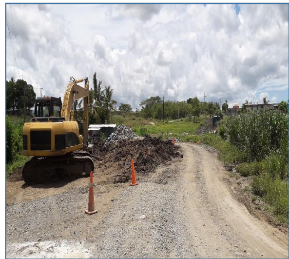
Photo 4 – No clear demarcation between the project site and temporary access road
