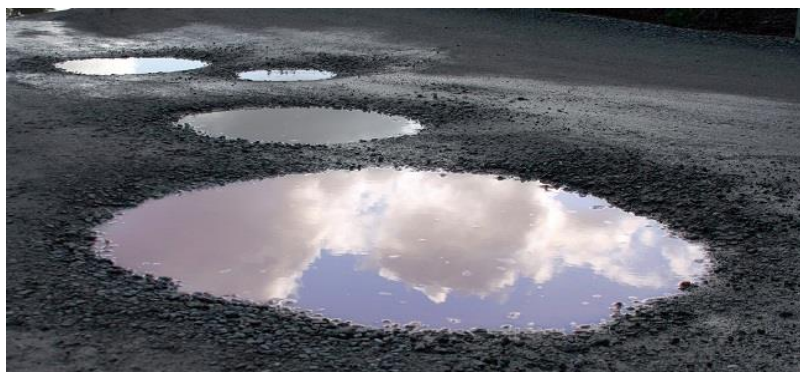
Potholes resulting from constant rainy weather conditions
