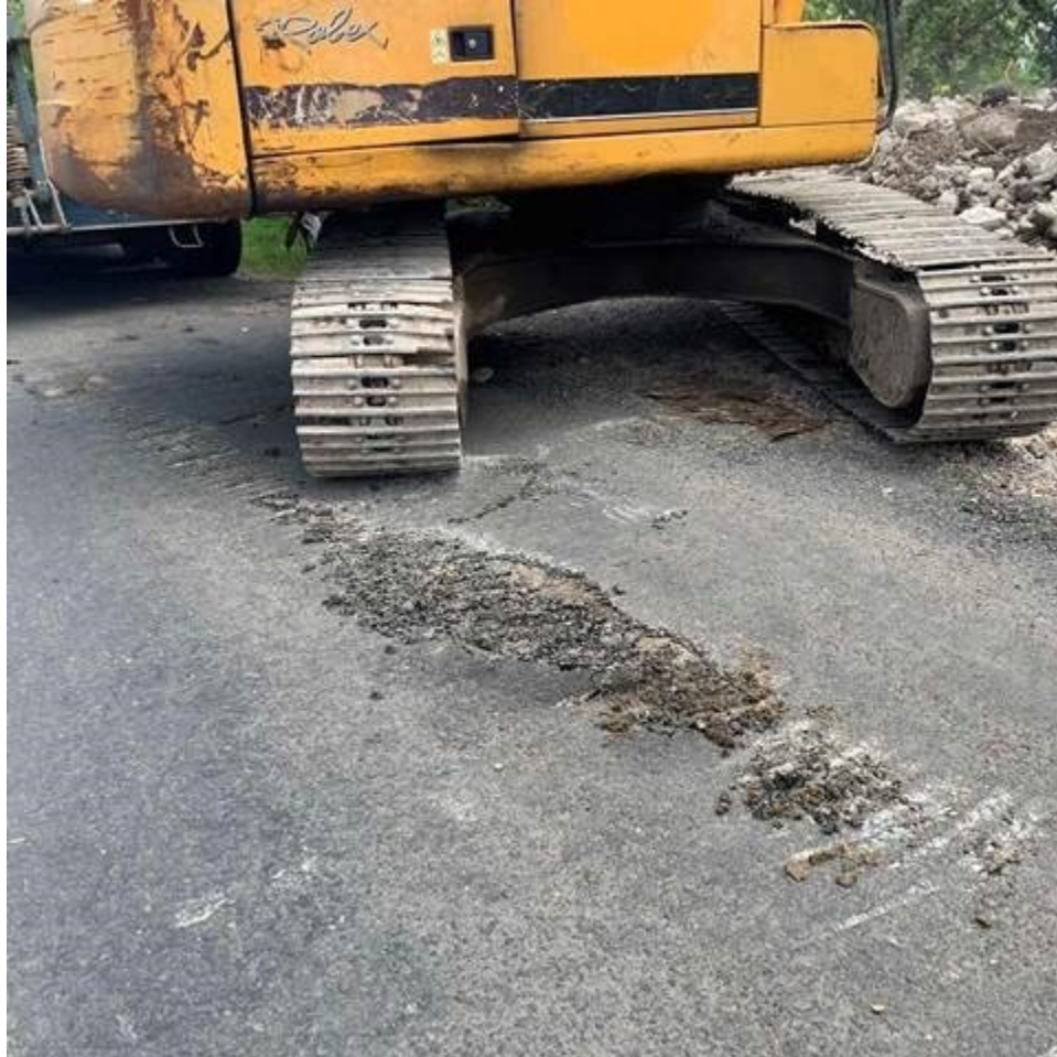
Picture Caption: Damaged seal while moving the excavator at Balabala Crescent in Nasinu
