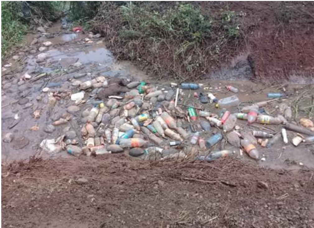
Blocked drain at Vaubasoga Road (Paras Point) Intersection with Vunivau Circular Road
