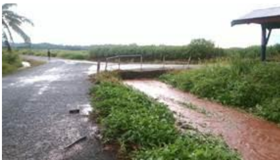
Vaubasoga Road – culvert blockage
