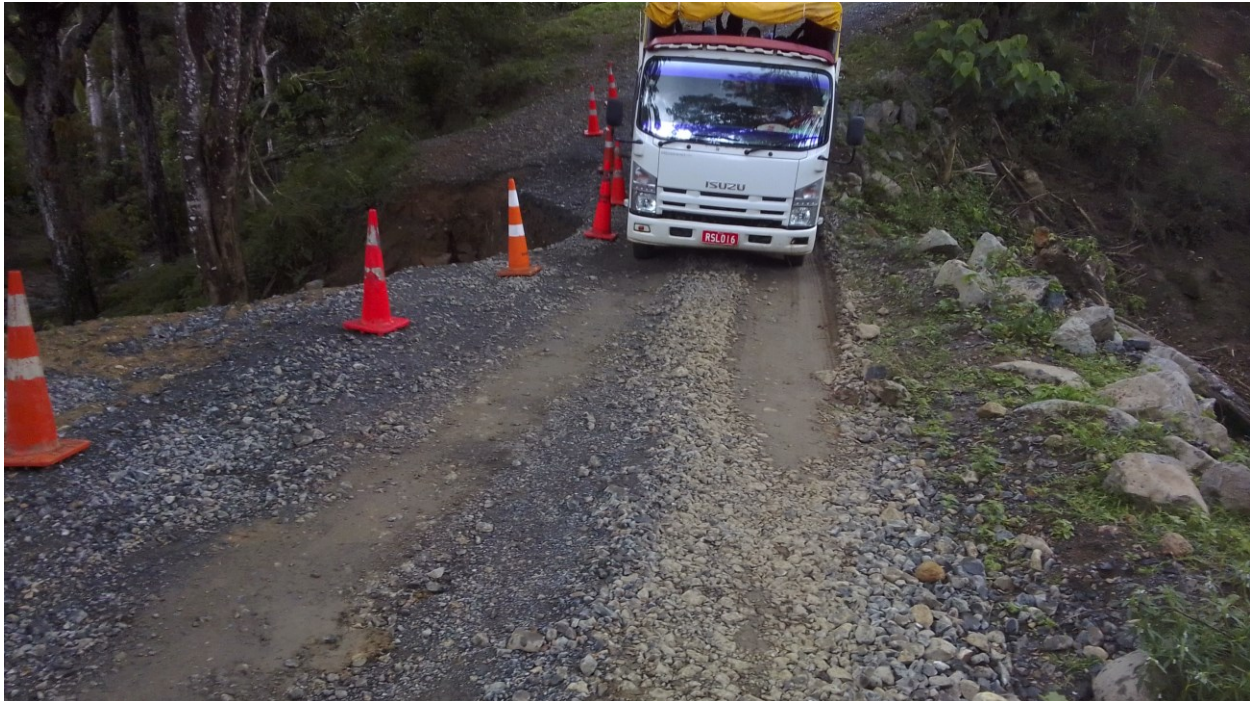
Under slip at Varialobo on Valley Road in Navosa.
