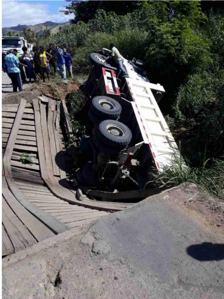
Image 2: The collapsed Maururu Bridge in Ba.
