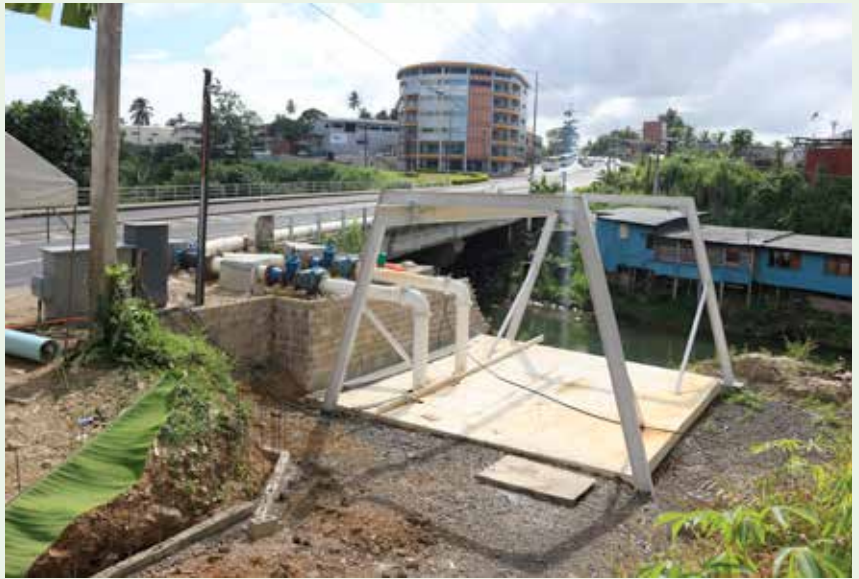
An example of shared road space is seen here. The replacement pipeline lies on top of the bridge.
