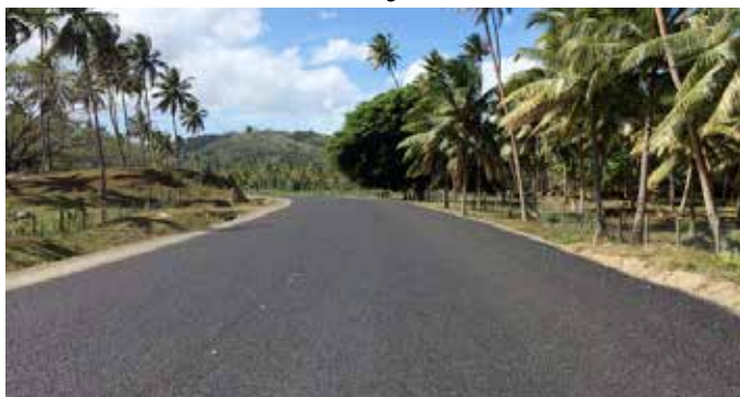
The work on the Buca Bay road will be completed this year.
