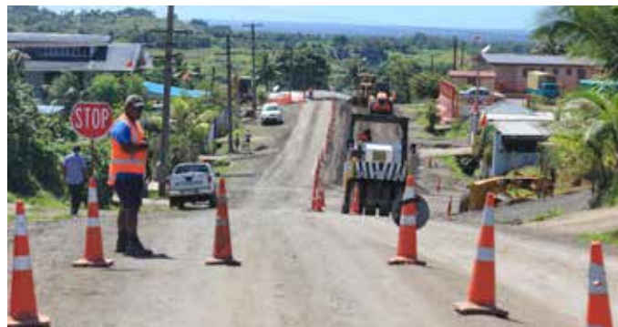
Upgrade works on Khalsa Road are the first for 2015 under this year's Road Recovery Plan.
