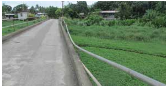
Vunivaivai bridge has been closed in the interests of public safety.
