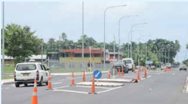
More improved street lighting in 2015 much like the improvements along Laucala Bay Road.
