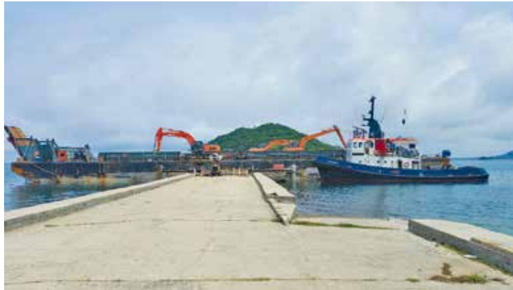
The Vanuabalavu jetty has been strengthened and is open in time for the holidays.
