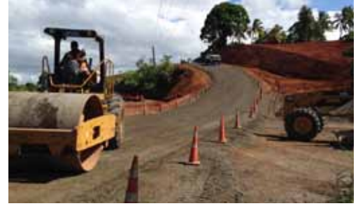
The slope has been cut away to reduce the slope and two lane access is now available.
